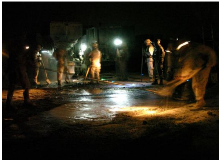
060520-N-9712C-010 Fallujah, Iraq (May 20, 2006) – Seabees pour concrete on a road repair project in Fallujah, Iraq. Naval Mobile Construction Battalion Four Zero (NMCB-40) is providing support to Multi-National Coalition Forces throughout Iraq. U.S. Navy photo by Photographer's Mate 3rd Class John P. Curtis (RELEASED)
