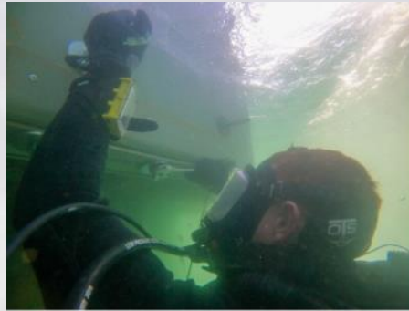
Construction Mechanic 2nd Class Zachary Reisinger, assigned to Underwater Construction Team 1 (UCT 1), secures bottom form work to a spire panel while working with Georgian divers
