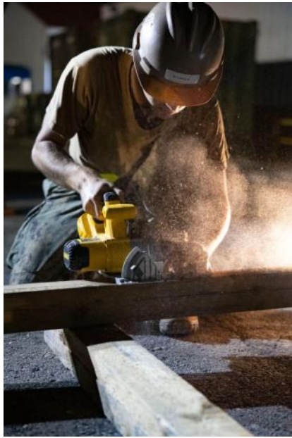
Builder Constructionman Apprentice Carson Bourque, assigned to Naval Mobile Construction Battalion 133 (NMCB 133), measures and cuts wood for palletization during a mount-out exercise on Camp Mitchell in Rota, Spain
