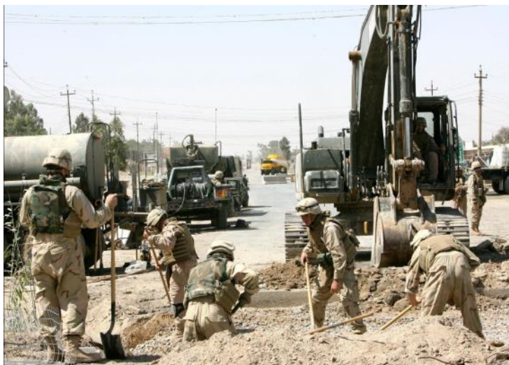
060616-N-9712C-010 Fallujah, Iraq (June 16, 2006) – Seabees prepare a site for the construction of a bridge. Seabees assigned to Naval Mobile Construction Battalion Four Zero (NMCB-40) were tasked with rebuilding a damaged bridge used heavily by Iraqi citizens. U.S. Navy photo by Photographer's Mate 3rd Class John P. Curtis (RELEASED)
