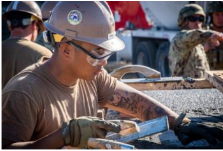
Seabees assigned to Naval Mobile Construction Battalion (NMCB) 5 place concrete during a field training exercise (FTX) onboard Naval Base Port Hueneme
