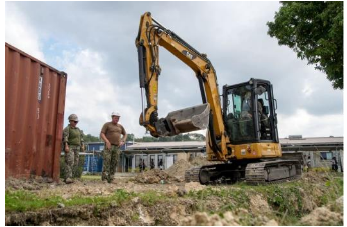
Equipment Operator 3rd Class Yue Zhao, from Los Angeles, Chief Equipment Operator Christian Ransomer, and Construction Mechanic Constructionman Apprentice Austin Loller dig a trench with an excavator at the National Referral Hospital in Honiara, Solomon Islands, during Pacific Partnership 2024-1. Photo by Cpl. Thomas Crivello.
