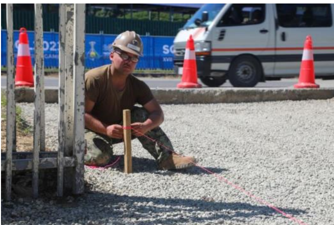
Builder 2nd Class Bryce Garcia sets up a concrete form at the National Referral Hospital in Honiara, Solomon Islands, as part of Pacific Partnership 2024-1. Photo by Cpl. Nathaniel C. Mansfield.
