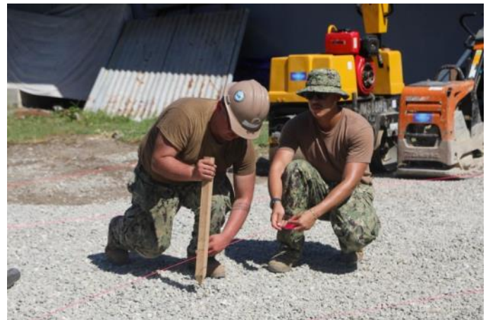
Utilitiesman 2nd Class Anthony Hellis, from Clayton, North Carolina, left, and Builder 2nd Class Bryce Garcia, from Camp Verde, Arizona, place string lines for concrete at the National Referral Hospital in Honiara, Solomon Islands, as part of Pacific Partnership 2024-1. Photo by Cpl. Nathaniel C. Mansfield.
