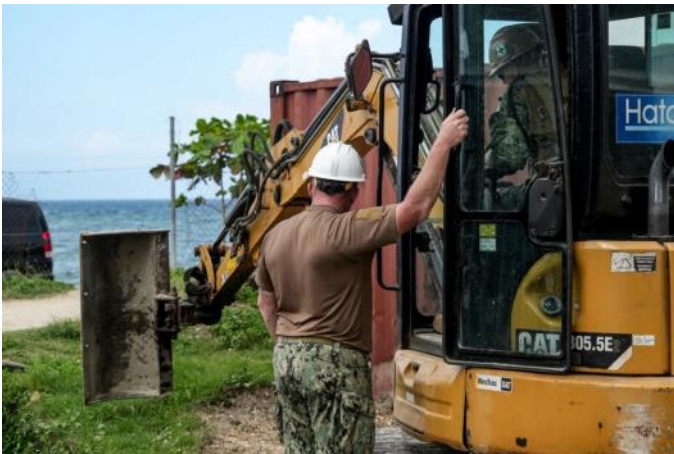
Chief Equipment Operator Christian Ransomer, from Dayton, Ohio, left, trains Construction Mechanic Constructionman Apprentice Austin Loller, from Fort Smith, Arkansas, on an excavator at the National Referral Hospital in Honiara, Solomon Islands, during Pacific Partnership 2024-1. Photo by Cpl. Thomas Crivello.
